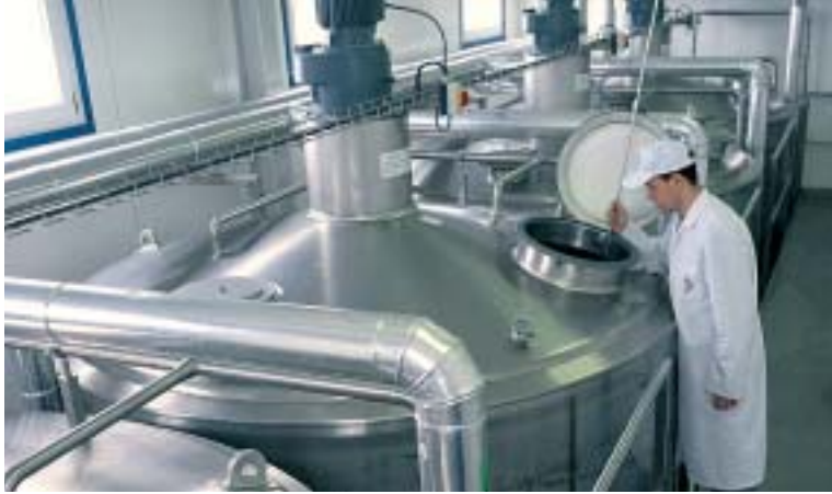
Whey crystallization tanks
