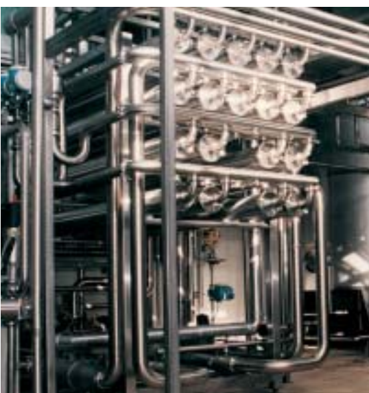
Ultrafiltration plant for whey
