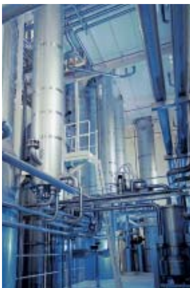
Falling film evaporator with thermal vapour recompression (TVR)
