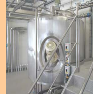
Wet mix tank
