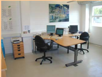
Process control room
