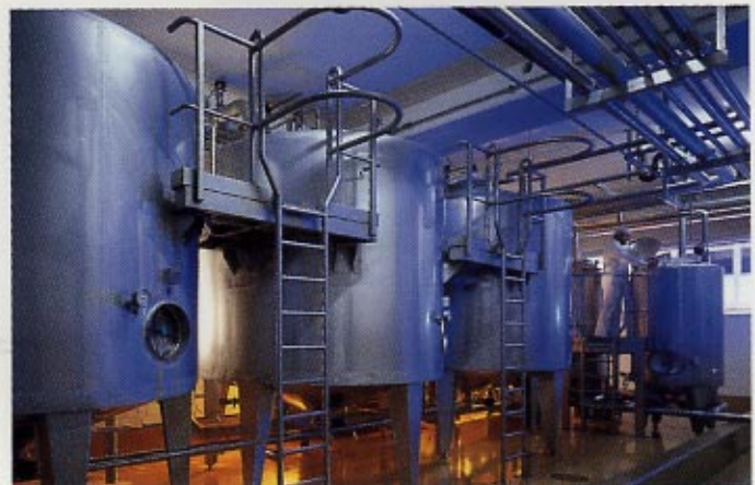
CIP kitchen comprising tanks for water, caustic soda, and acid.
