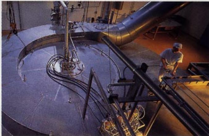
Preparing the feed line and high pressure nozzle atomizer for CIP cleaning. The operator places the nozzle lances in a tray, then attaches the pressure hoses before the cleaning cycle is started.
