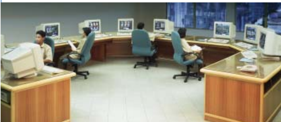
Process control room
